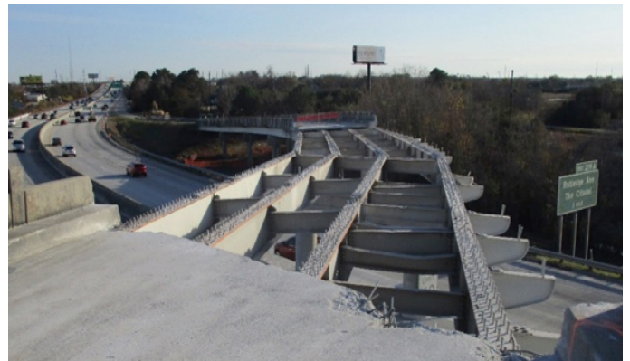
Photo Above – Having removed all of the concrete parapet walls and deck on the former I-26 Exit 218 ramp from Spruill Avenue to I-26 Eastbound, crews will work at night in early January to remove the remaining ramp components over I-26.
