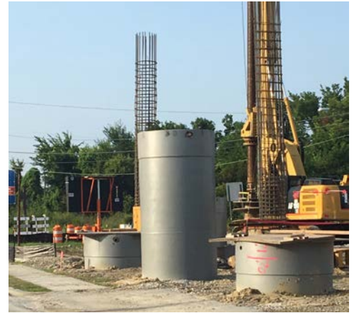
Photo Above: Drilled shaft casings are required to be painted for the Port Access Road mainline to resist corrosion.
