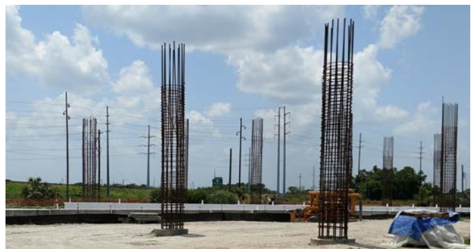
Photo Above: Rebar column cages stand in anticipation of concrete to be placed in July.
