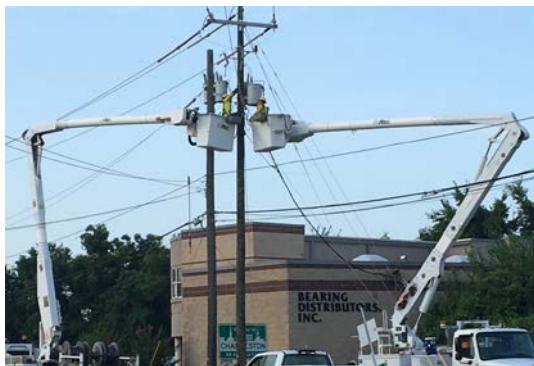
Photo Above: Utility relocation continues. In this photo an electrical contractor moves service from one pole to another.
